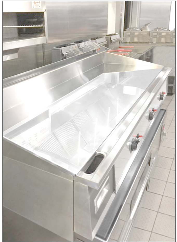
72x30 Keating Miraclelean® gas Griddle being installed at the Burgerhaus in Indianapolis, IN.
